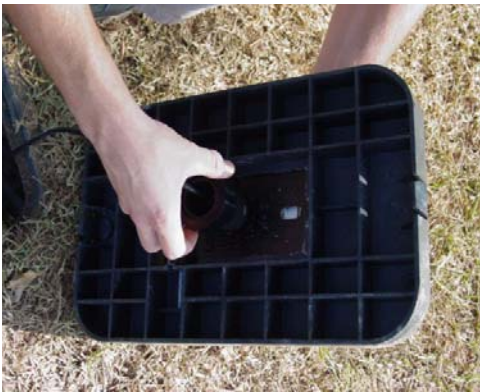
Figure 14 Feeding Antenna Cable
